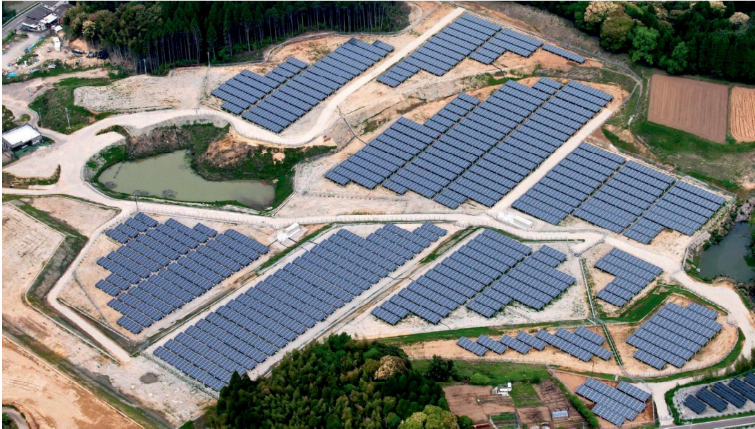
Fig.10 Largest solar power plant of India at Kamuthi [10]
