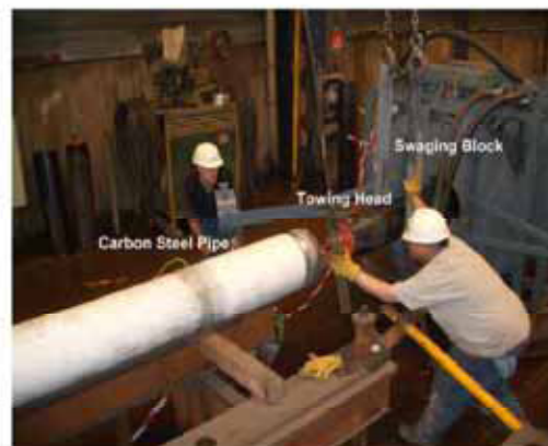
Fig No. 2 Reduced Plastic liner pulled from swaging block via a towing head about to go into the pipe
