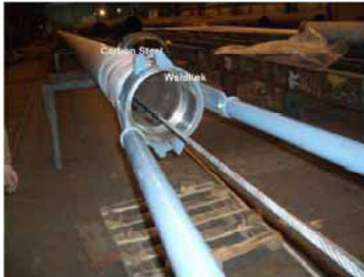
Fig No. 3: Plastic liner pulled through the steel pipe with the Weld link welded to the end of the stalk
