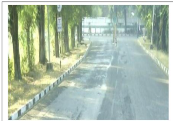
Image No 9 :In this portion Emulsion is not Sprayed Properly so, that portion is also damaged.
