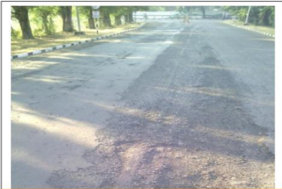
Image No 2 : After 3 years it is observed that the portion where Emulsion is sprayed is well good and on the other side where it is not done (at that time it was in good condition) is damaged which require maintenance (overlay).
