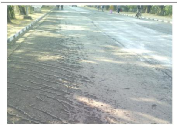
Image No 7 :Patch repairing work done in Right Sideportion where preventive measures has not done.
