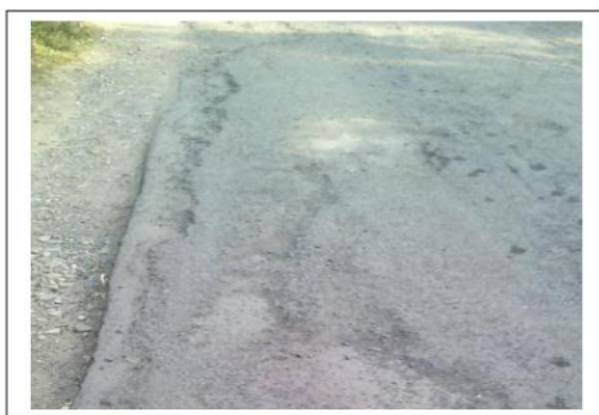
Image No 8 :Overlay in PQC (Damaged)
