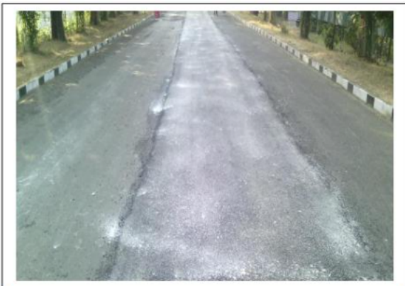
Image No 3 : In Dec 2014 Patch repair is being required & done in middle portion at portion where preventive measures has not done. Latitude 23.135624 Longitude 79.912663.
