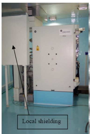
Fig. 1 Medical Cyclotron in indigenously designed bunker with ~2 metre thick concrete vault walls and ~1 metre haematite concrete roof. Local shield shielding built to reduce neutron streaming towards vault maze.
