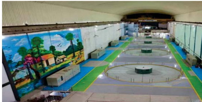
Fig. 9 Pump House equipped with 4x134.4 MW Pumps
