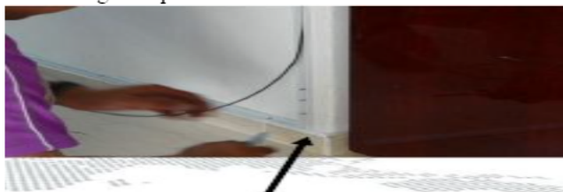
Sharp bend Fig.1b Optical cable with heavy bends
