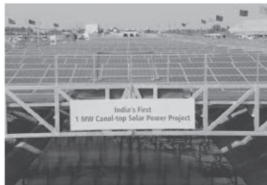
Fig. 4: Canal-top Solar PV Power Project (1MW)
