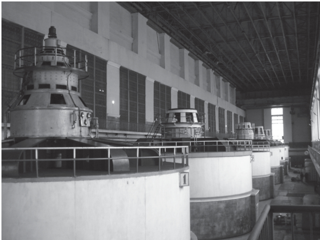
Fig. 3 View of power house with one old and other new generating units
